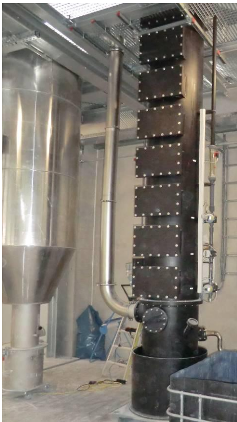
Fig. 5: Scrubber for the removal of methanol
