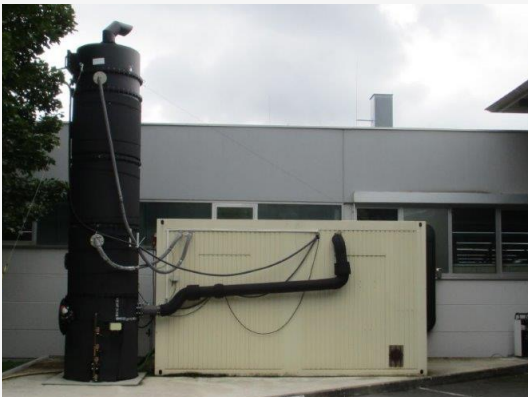
Test plant for process qualification
