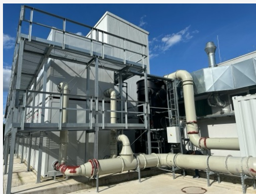
Industrial plant for 10.000 m 3 /h exhaust air
