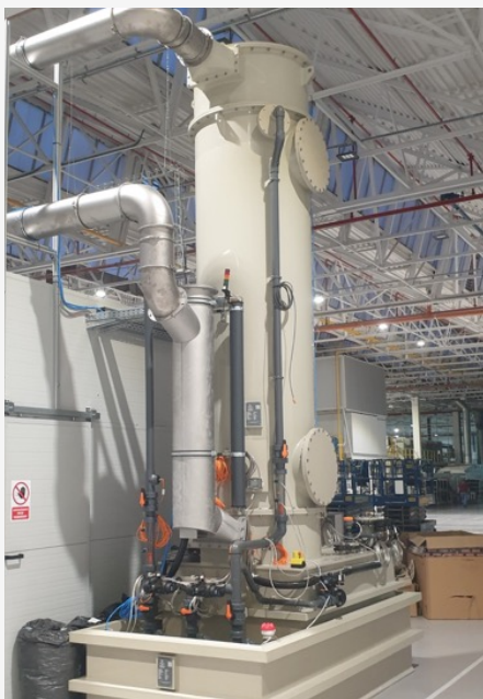
Plant for 1 x 2500 m 3 /h, PP
