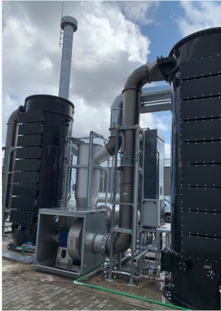
Plant for 2 x 7500 m 3 /h, el. conductive PE
