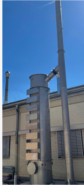
Plant for 2500 m 3 /h, stainless steel
