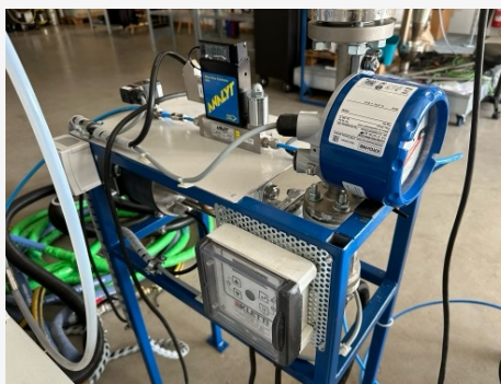
Gas and steam supply
