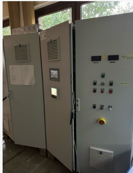
Power supply including Process control unit
